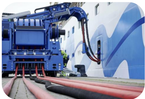
ON SHORE POWER SUPPLY (OPS)
