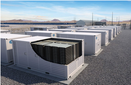
Local or Centralised Battery Storage
